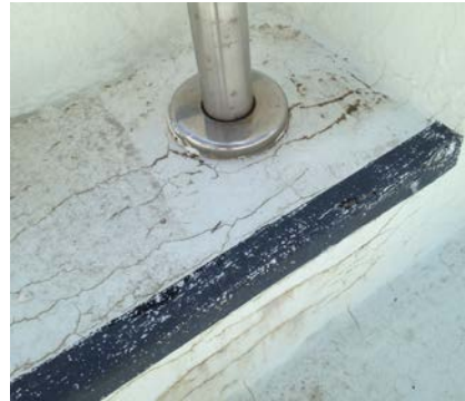
Fig 4. Capped Skimmer Line
