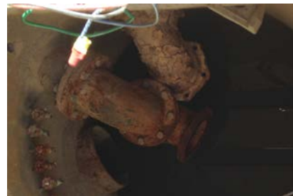
Fig 7. Corroded drain pipe
