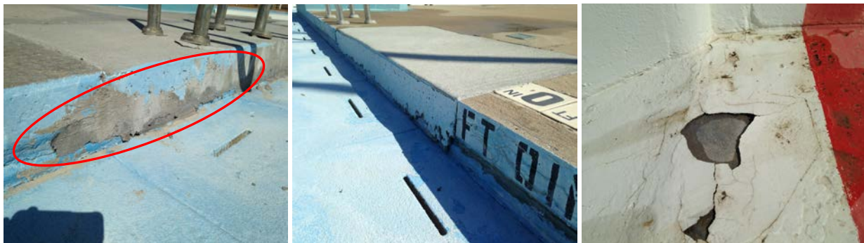
Fig 2. Deteriorated gutter/deck joints and delaminating concrete
