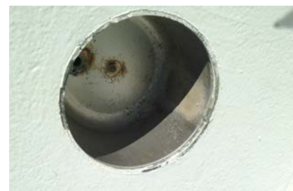
Fig 3. Missing pool light
